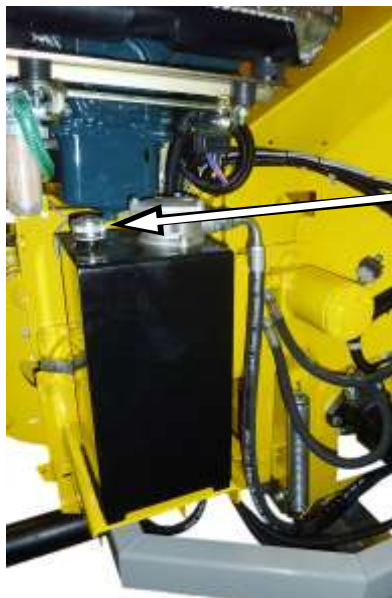
LEVEL IN THE HYDRAULIC TANK
